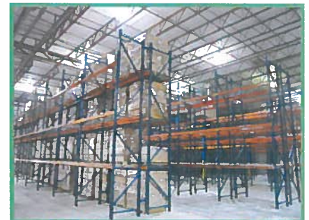
Pictured above: The newly rebuilt Delta facility, featuring the new racks that will soon be completely filled with Asset Management product.
